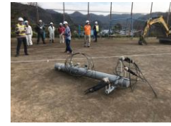
collapsed utility pole
